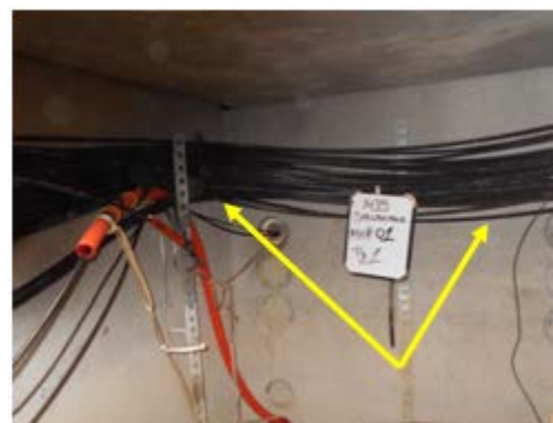
Unacceptable – More than 3 wraps
